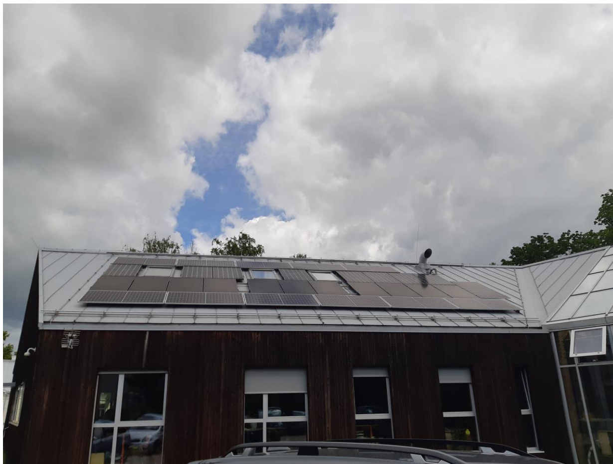
Figure 8: PV-park at Lille str. 10
