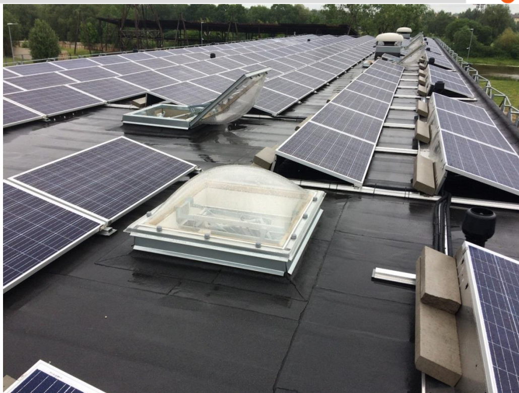
Figure 5: Solar panels on the cooling plant roof
