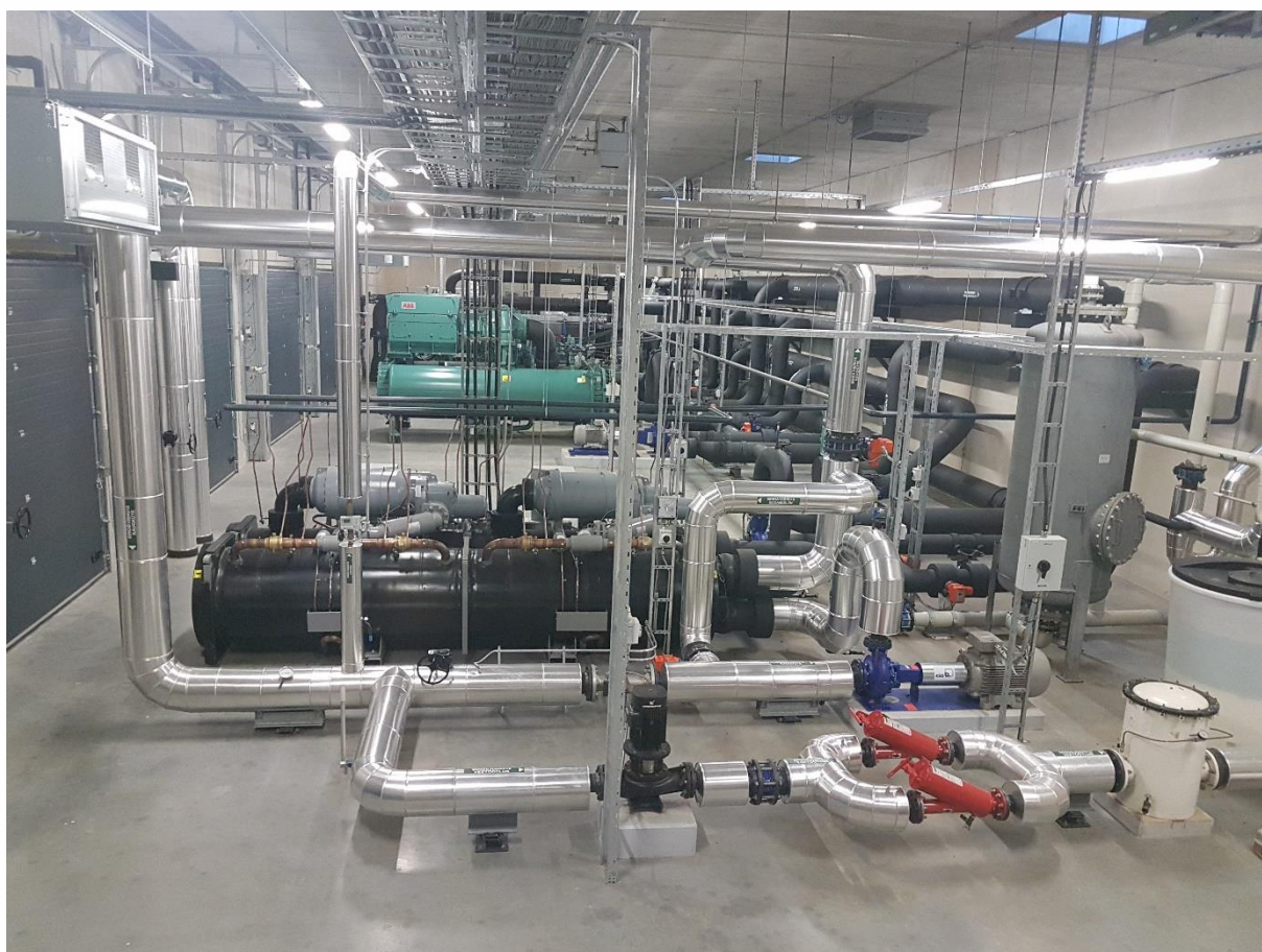
Figure 1: Internal view of cooling plant
