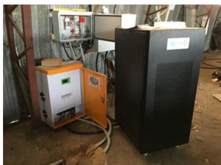
Figure 11: Solar combined box (left) and inverter (right)
