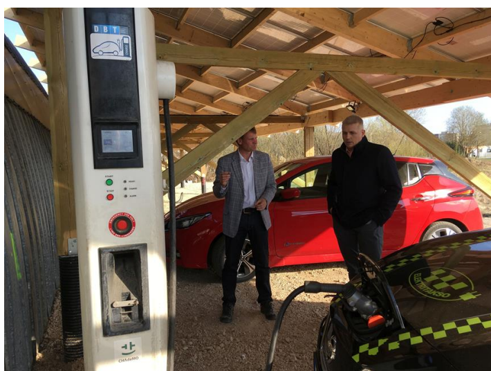
Figure 7: EV-battery re-use system in operation in Tartu at Takso OÜ workshop
