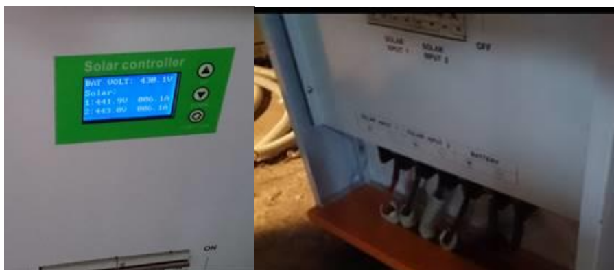
Figure 12: Solar combined box
