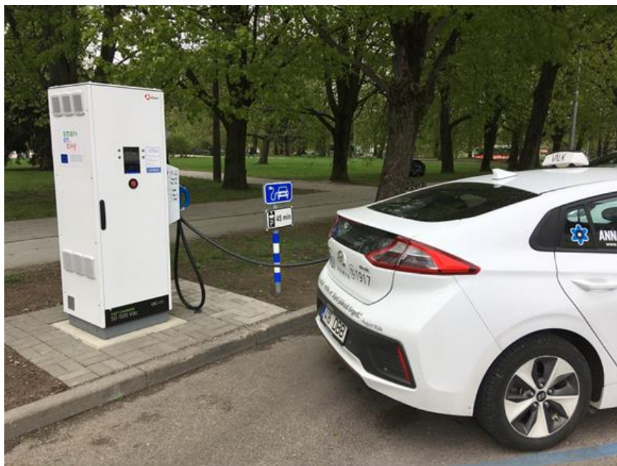
Figure 1: EV-charger in Uueturu street
